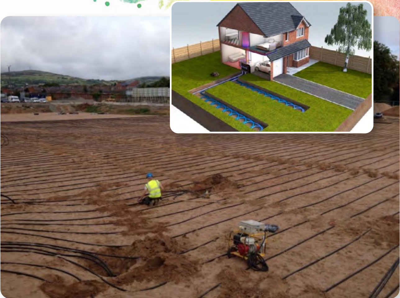
Fig. 5: Photograph showing plastic pipes laid in shallow trenches underground for a horizontal closed loop geothermal heating system alongside a three dimensional representation of the system.
